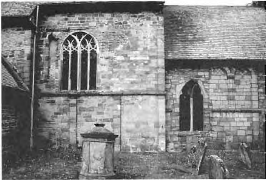
Figure 1: The south elevation of the chancel at the church of St Mary, Dymock, Gloucestershire, showing complex phases of masonry.
