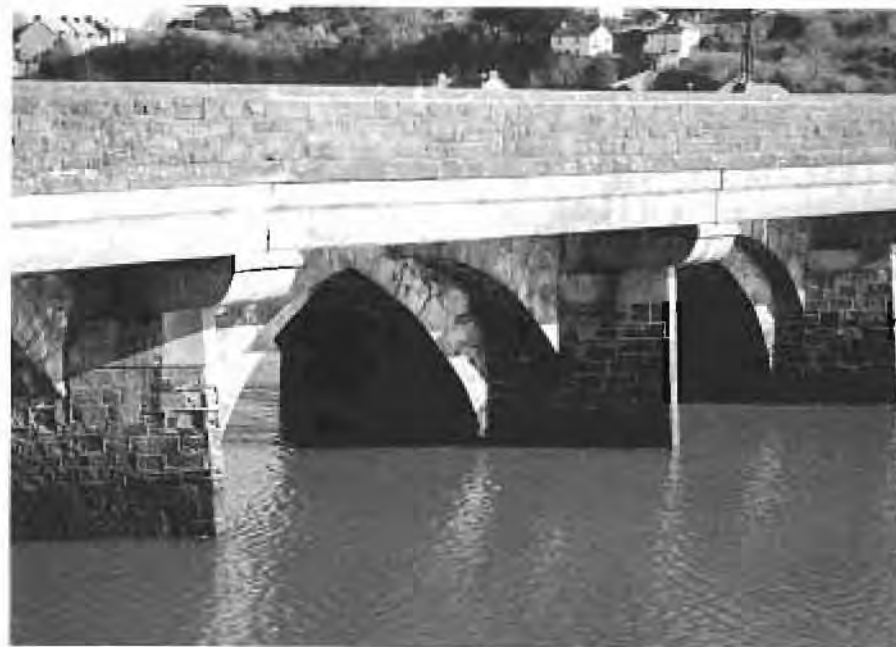
Bideford long bridge: upstream face showing original Gothic arches; 1795-1810 widening by segmental arches between the cutwaters and 1924-1925 widening in reinforced concrete.
