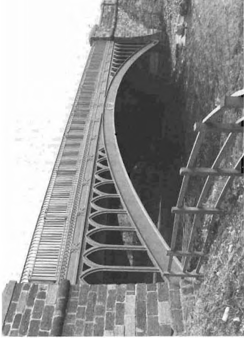
St Saviour's Bridge in Ottery St Mary. Downstream view.
