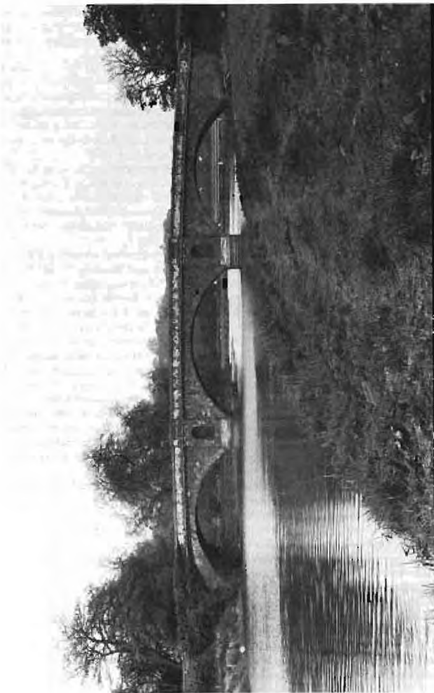
Cowley bridge, River Exe, 1814, Carrying Exeter to Crediton road. Photo: A B George.
