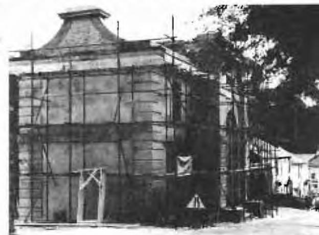
Old Police Station and Debtors' Prison at Tiverton in process of restoration by the Devon Historic Buildings Trust.
