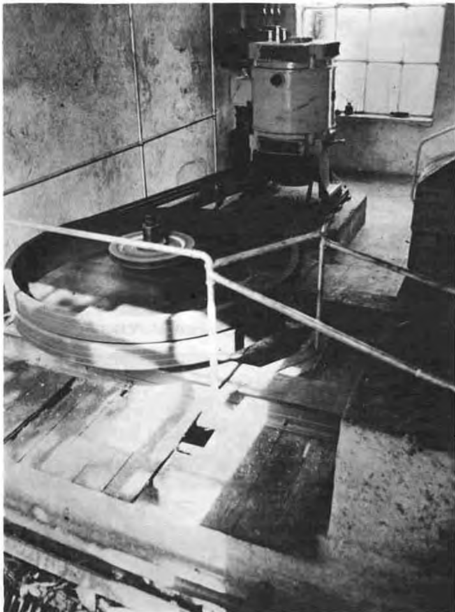
Plate C The present equipment of the Chagford station: the turbine is below the floor and directly coupled to the flywheel; the generator (26 kW, 420 volt, 3-phase, made by the Electric Construction Co.) is driven by belts from the flywheel. (Photo by D.G. Tucker)
